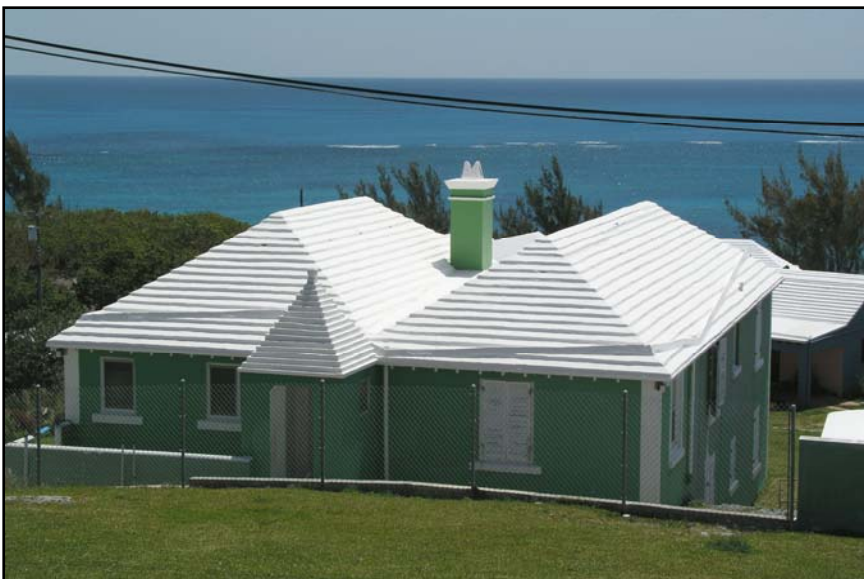
Figure 4. Roof catchment. Gutters or "glides" slope down to leader pipes, which transfer rain water to the tank. Approximately 80% of this roof is guttered, which is the typical percentage.
