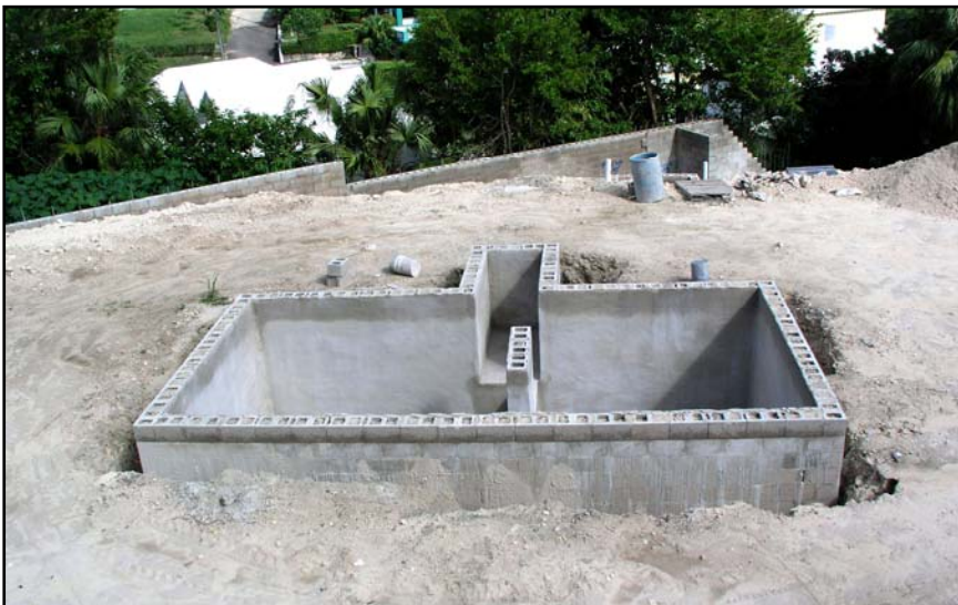
Figure 3. Rain water storage tank. 24 ft x 12ft x 8ft (deep), with a capacity of approximately 14,500 Imperial gallons, which is typical of a modern household tank.
