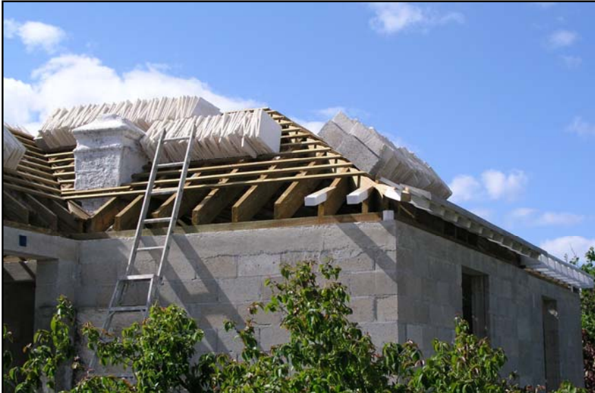
Figure 2. Bermuda roof under construction. Shown are the timber frame and the limestone slates ready for positioning.
