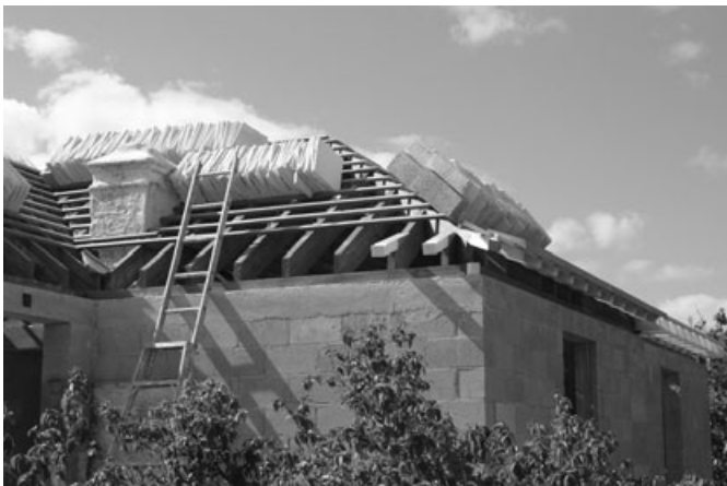
FIGURE 2. Photograph Showing the Construction of a Bermuda Roof. A heavy wooden framework of rafters is constructed to support “slates” of Bermuda limestone which are shown stacked up ready for positioning. They will be overlapped with an intervening bed of cement-and-sand mortar.
