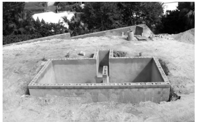
FIGURE 4. Photograph Showing Construction of a Bermuda Water Tank. This rain water storage tank constructed of concrete block is located in an excavation which will be covered with the floor slab of a future house. The size is typical for Bermuda, measuring 7.3 \text{ m} \times 3.7 \text{ m} \times 2.4 \text{ m} (deep) with a capacity of 65 \text{ m}^3 .
